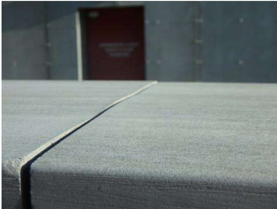
Figure 48 – Matt top surface of the wall feature in front of Pymont Wharves 8 and 9.
