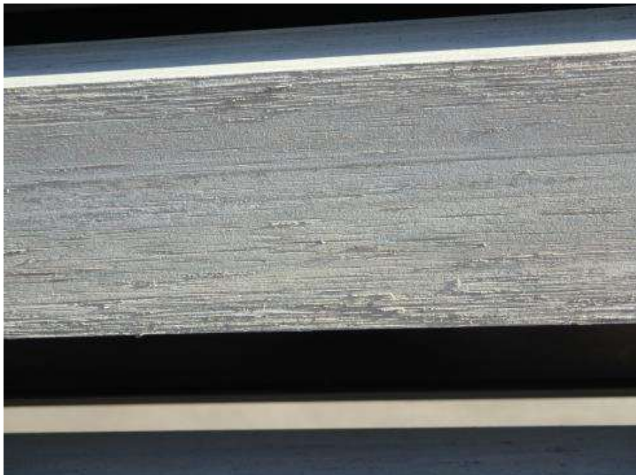
Figure 51 – Close-up of (a rare instance of) minor surface peeling in the side surface of the wall feature in front of Pyrmont Wharves 8 and 9.
