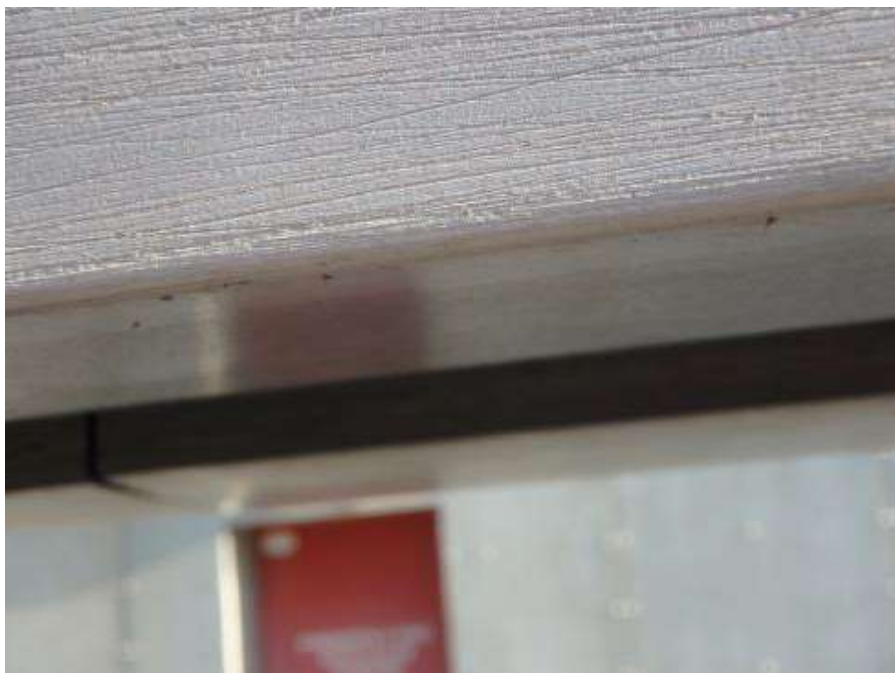
Figure 49 – Shiny under surface of the wall feature in front of Pymont Wharves 8 and 9, revealed by reflection of a door.
