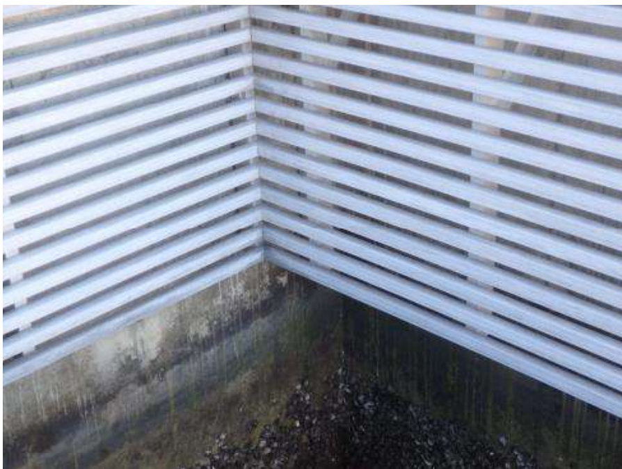
Figure 42 – View of the slatted covering on the lower portion of the building walls at Pyrmont Wharves 8 and 9 showing its close proximity to the high water level.
