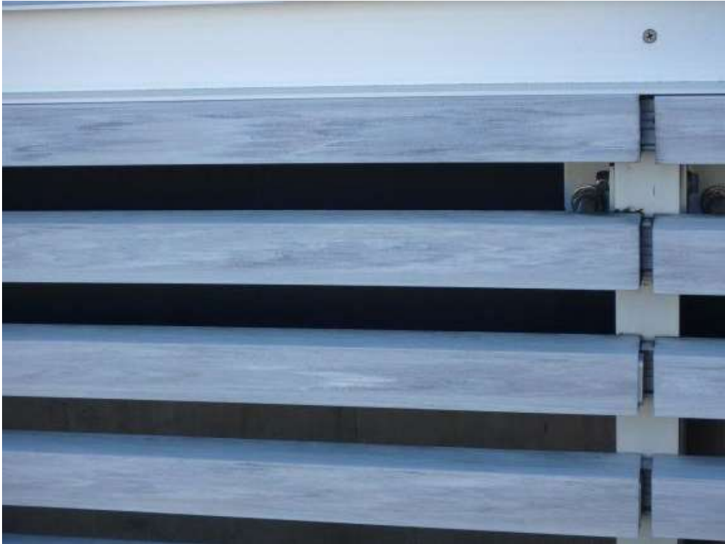
Figure 45 – Close-up of the slatted covering expansion joints on the lower portion of the building walls at Pymont Wharves 8 and 9.
