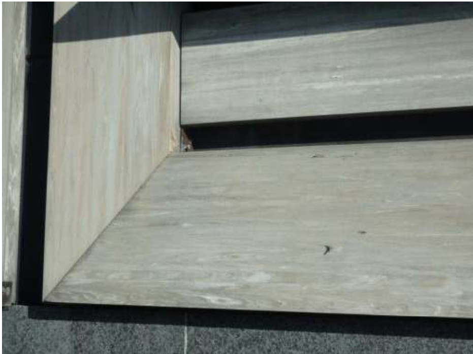
Figure 37 – Detailed view of 45° joints in a vertical section of the Wild Life Sydney Zoo Façade.
