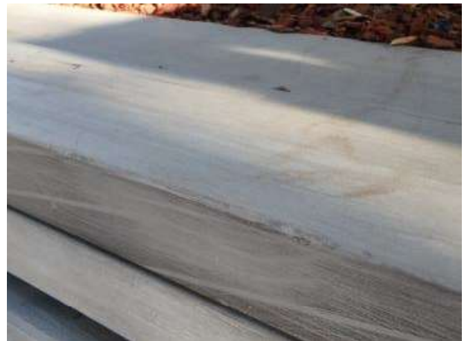
Figure 56 – Corner scrape in the East planter surround in front of Pymont Wharves 8 and 9.
