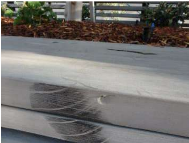
Figure 55 – Tyre marks and impact indentation in the East planter surround in front of Pymont Wharves 8 and 9.
