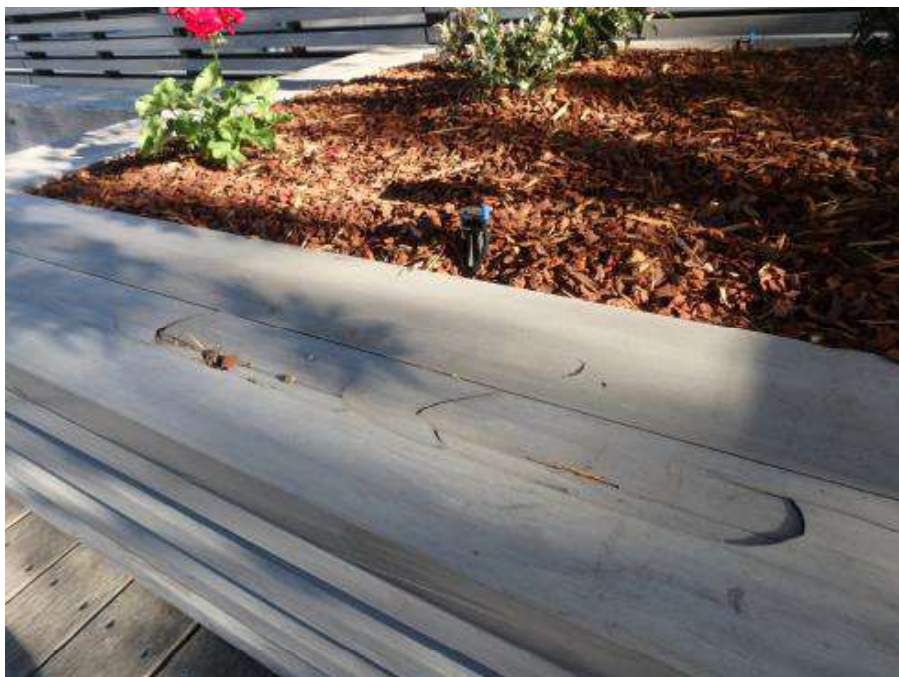
Figure 53 – Damage in part of the East planter surround in front of Pymont Wharves 8 and 9.
