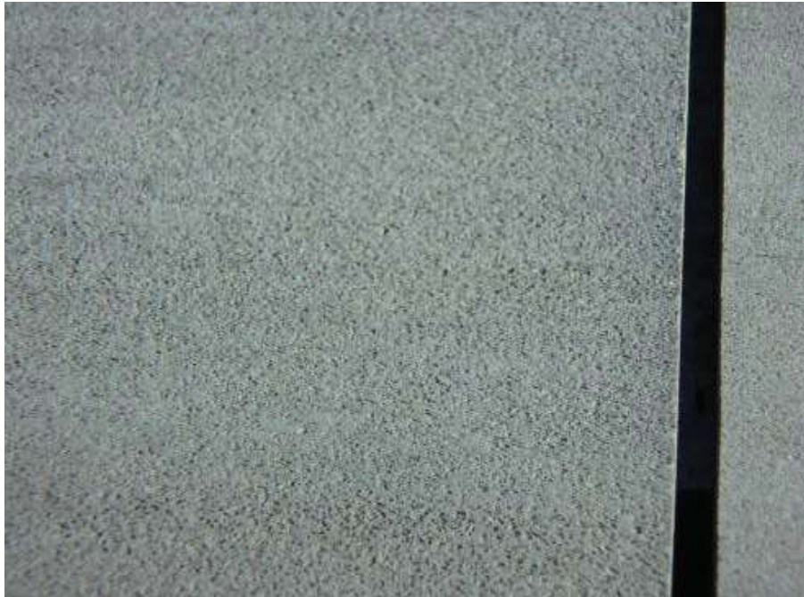
Figure 50 – Close-up of pits in the top surface of the wall feature in front of Pyrmont Wharves 8 and 9. The plank gap is ~5mm wide.
