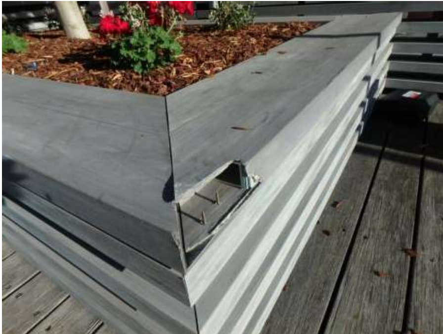
Figure 54 – Corner damage in the West planter surround in front of Pymont Wharves 8 and 9.
