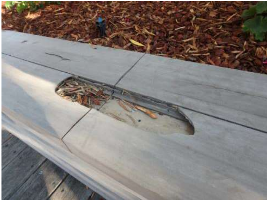
Figure 52 – Damage in part of the East planter surround in front of Pymont Wharves 8 and 9.
