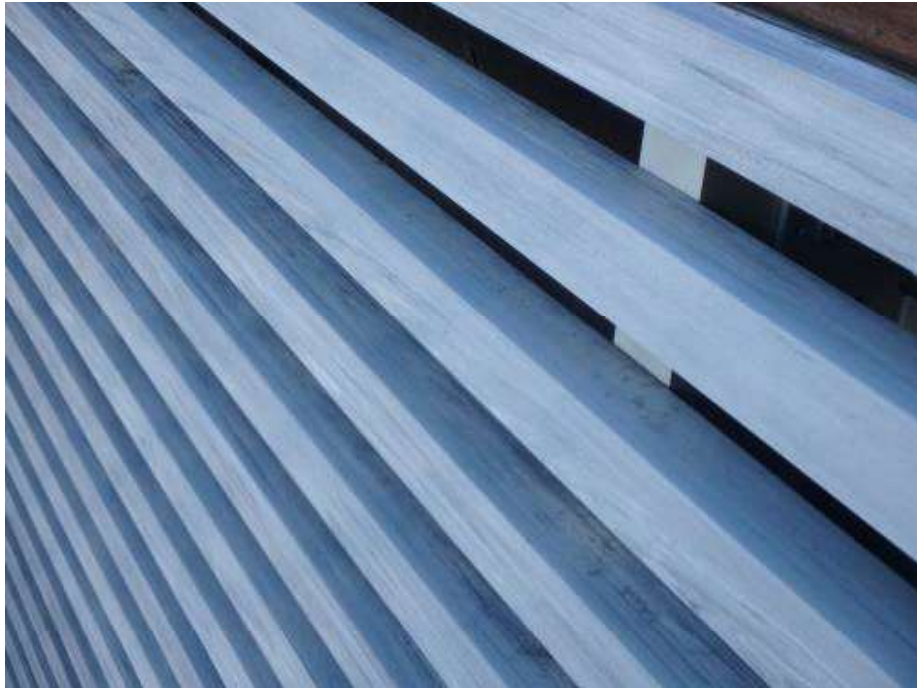
Figure 43 – Close-up of the slatted covering on the lower portion of the building walls at Pymont Wharves 8 and 9.
