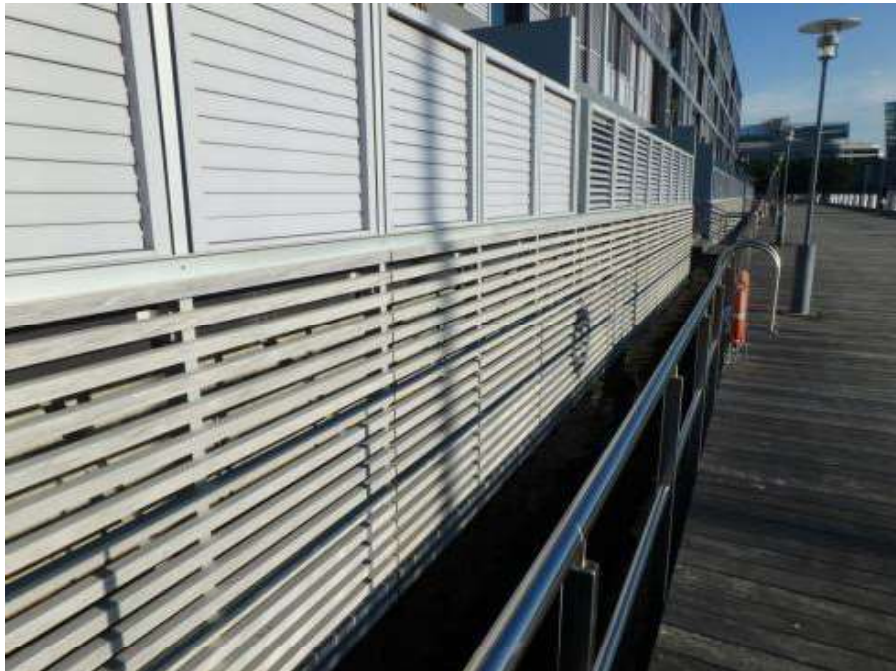
Figure 41 – General view of the slatted covering on the lower portion of the building walls at Pyrmont Wharves 8 and 9.
