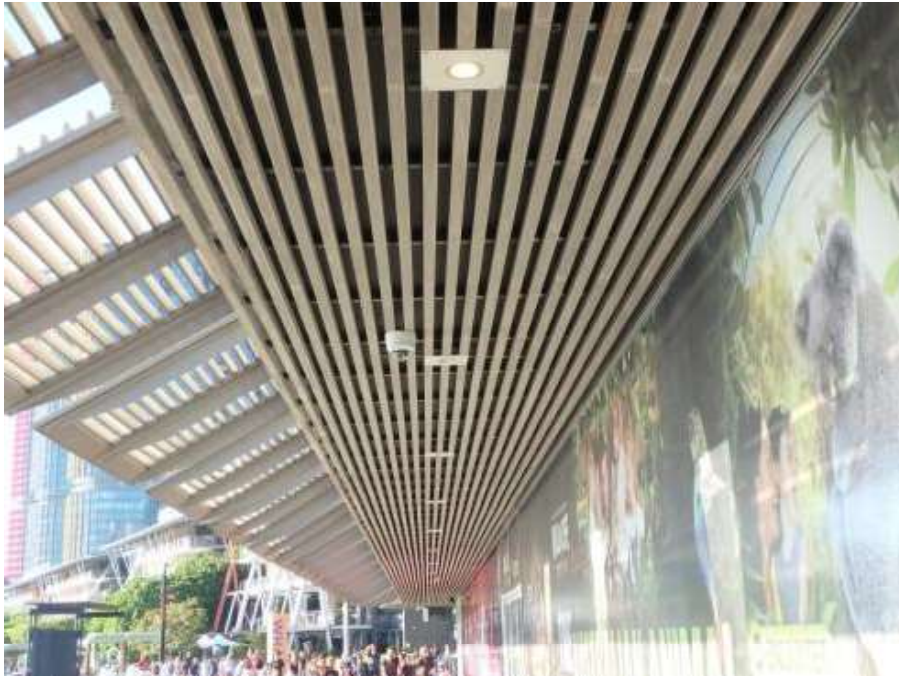
Figure 39 – General view of the slatted ceiling at the Wild Life Sydney Zoo
